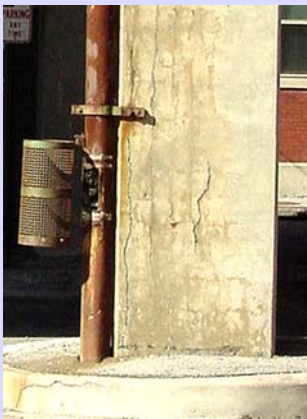
Deteriorating concrete piers.
