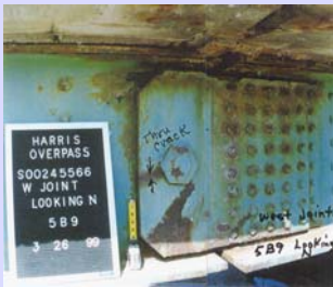
Cracks in steel plates, rusting girders.
